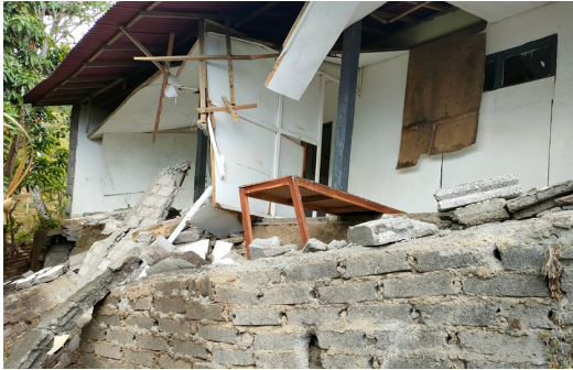
The 2 rear classrooms that collapsed
